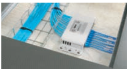
Cablofil wire mesh cable tray and area distribution box
